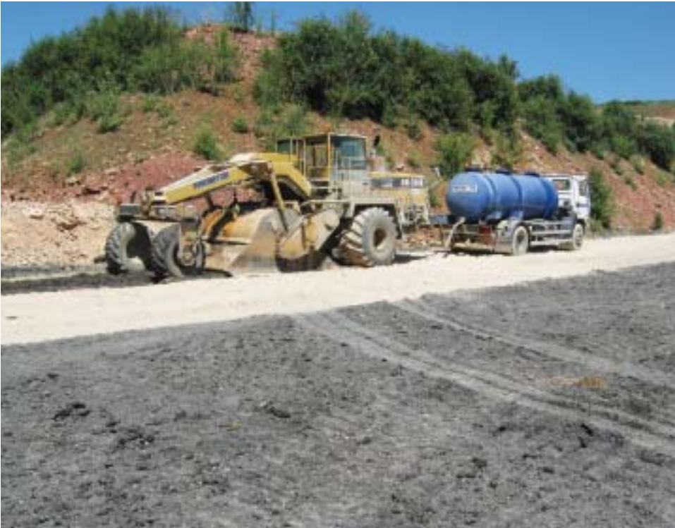
Fig. 3. Rotavator plant mixing a layer of kiln dust and colliery spoil prior to compaction for the formation of the basal perimeter layer
