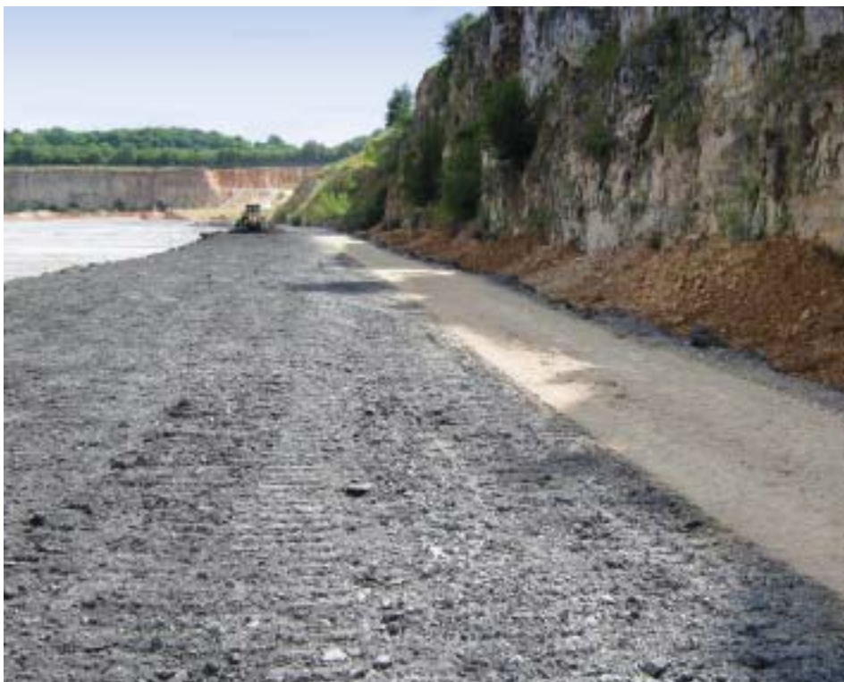
Fig. 2. Mixing of kiln dust and colliery spoil prior to compaction to form the base of the perimeter side wall
